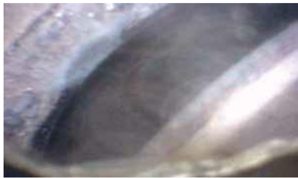
Almost too late for this seat. You can see where erosion has begun.
